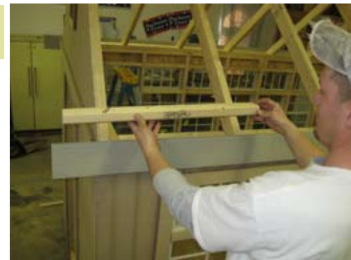
Purlins will be installed on top of trusses for Sunsky to set on.
